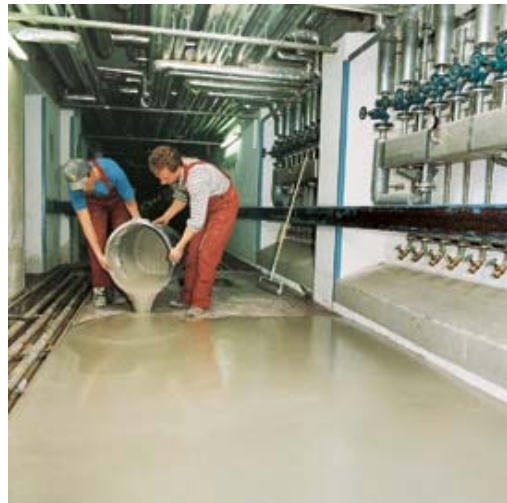
Floor levelling compound covering the entire area with self-levelling Mastertop 540 for direct usability.
