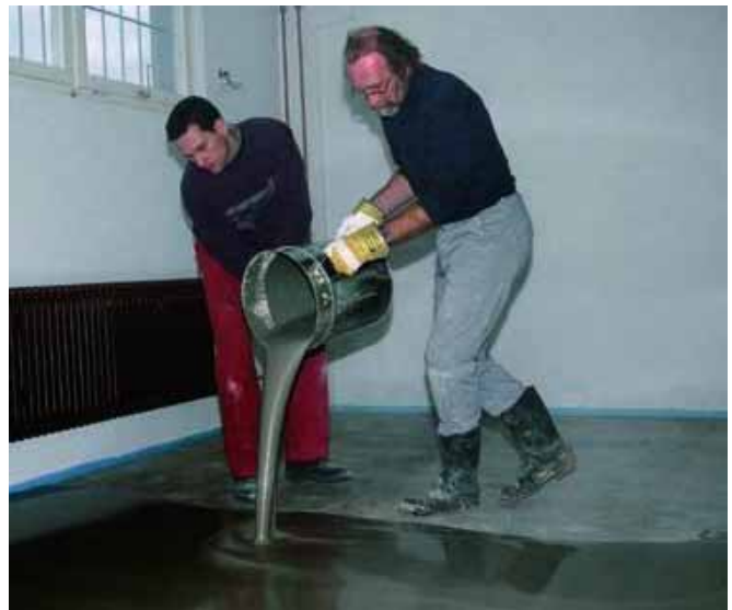
Efficient levelling of floors with PCI Periplan prior to laying top coverings.
