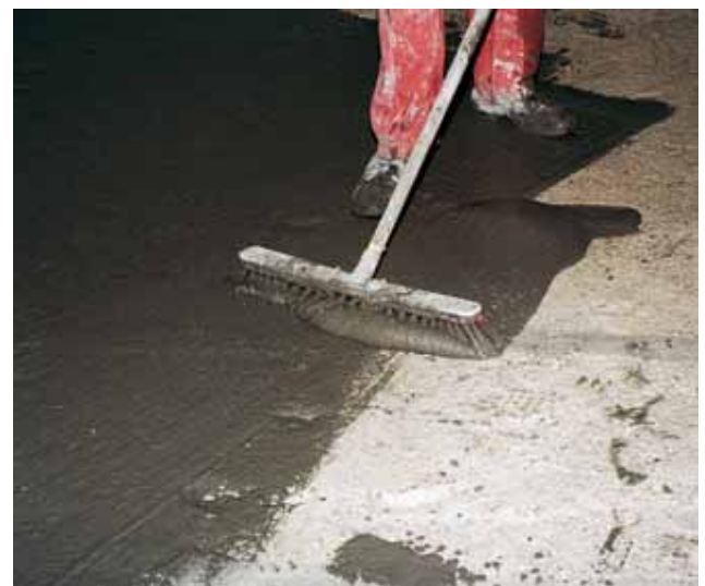
PCI Repahaft is brushed on to the substrate. After this the screed mortar is immediately applied on to the fresh bonding agent.
